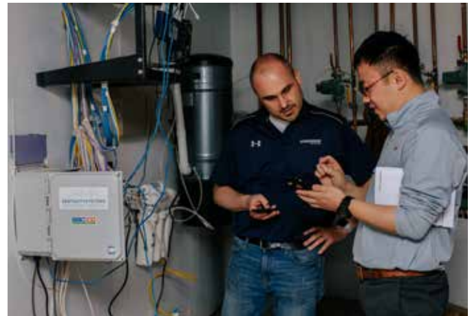
Ferguson's Karol Tomaszewski and Fujitsu's Xiaofan Yang work on system controls during commissioning.
